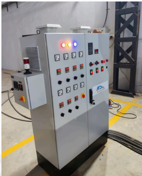
FULLY AUTOMATD PANEL BOX WITH VFD CONTROLLING SYSTEM
